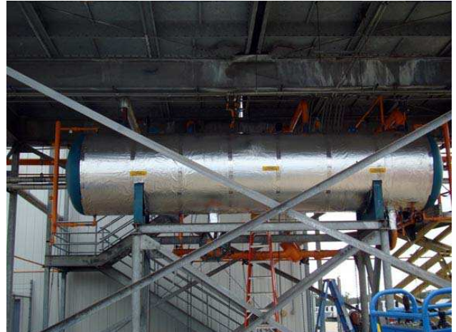
WEATHER PROTECTED VESSEL
